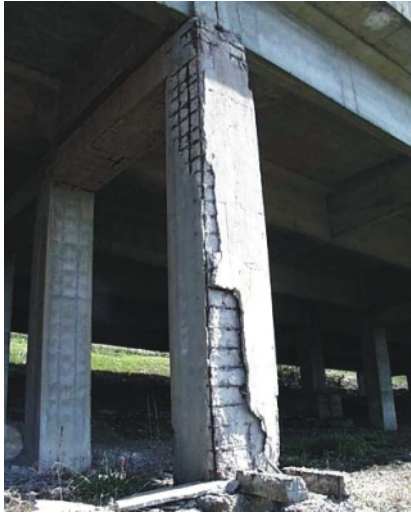
Fig. 5 Concrete bar cover damage
