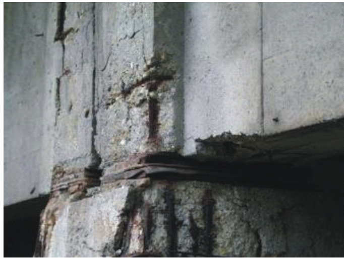
Fig. 6 Existing bearings degradation
