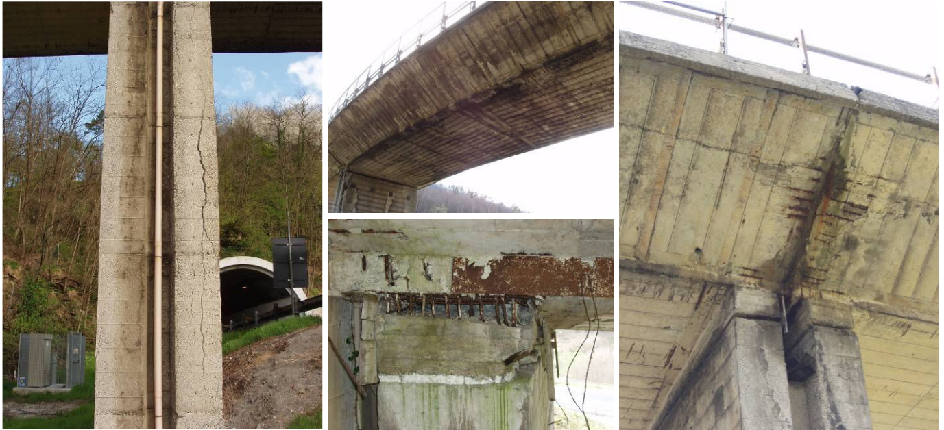
Fig. 4. "Carrodano" viaduct: structural details and examples of local damage
