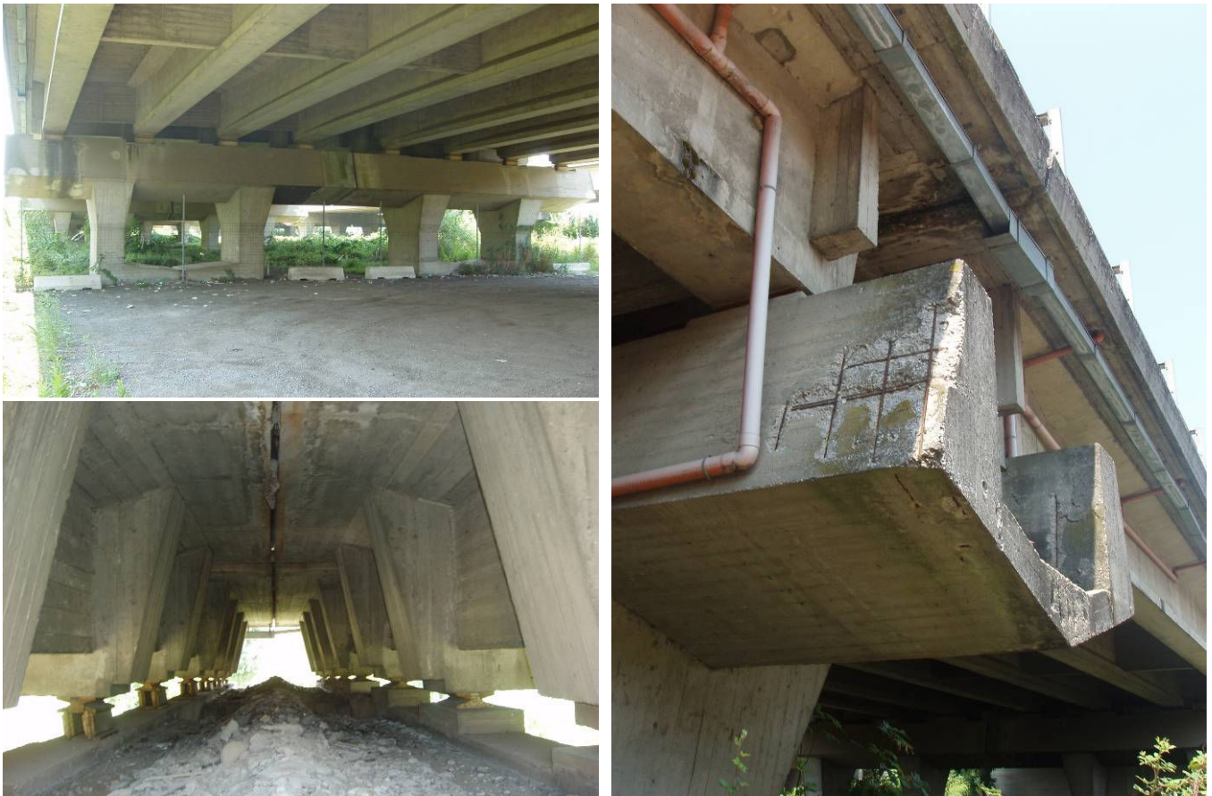
Fig. 8. "Torre del Lago" viaduct: structural details and examples of local damage
