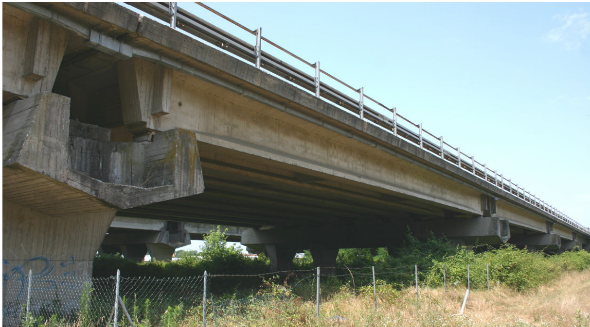
Fig. 6 Partial view of "Torre del Lago" viaduct (neighbouring the Viareggio town, Tuscany, Italy)
